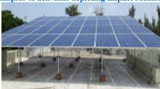
Solar roof top system at Forestry UG Boys Hostel, Navsari
