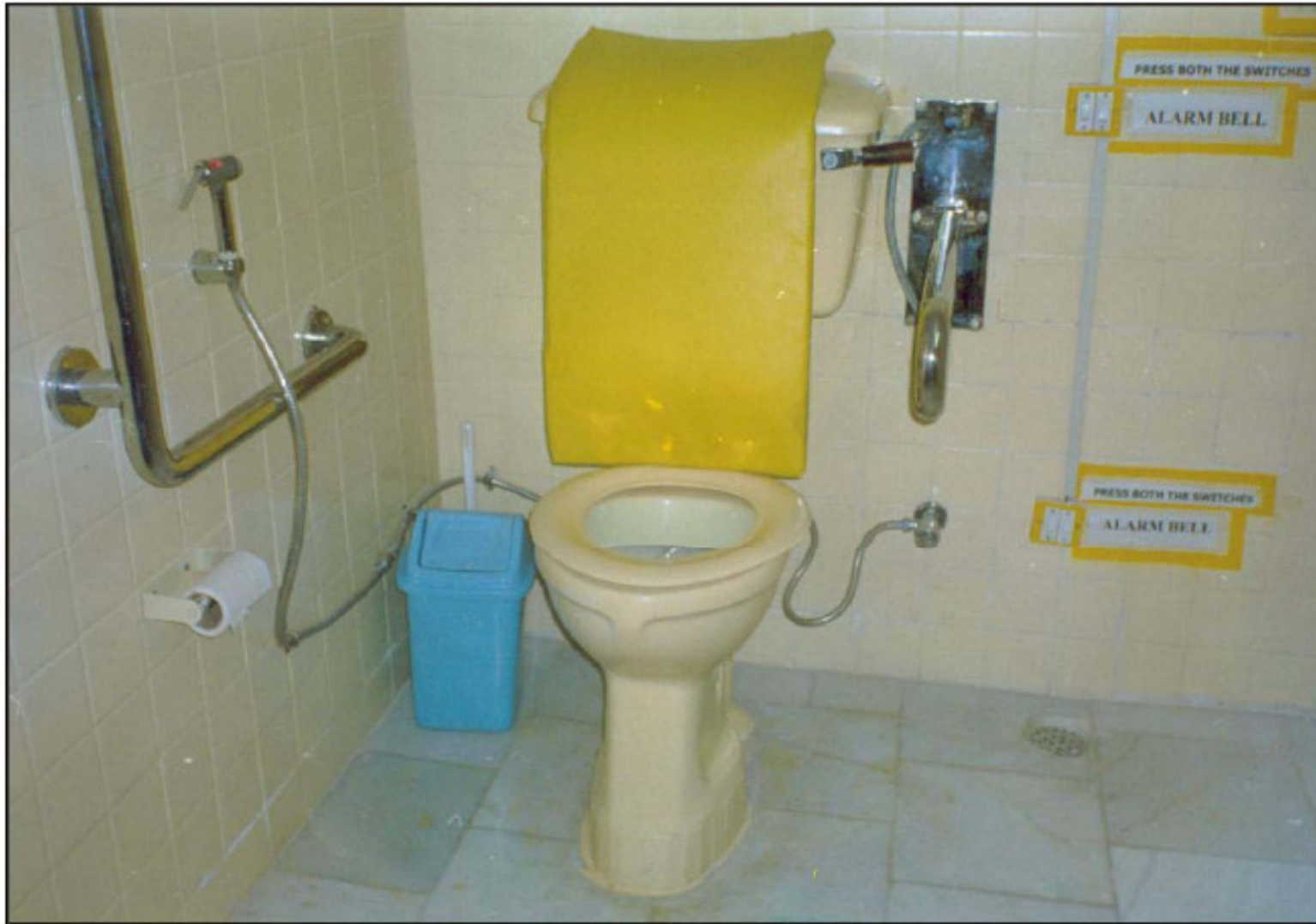
Good example of Grab bars in accessible toilet
