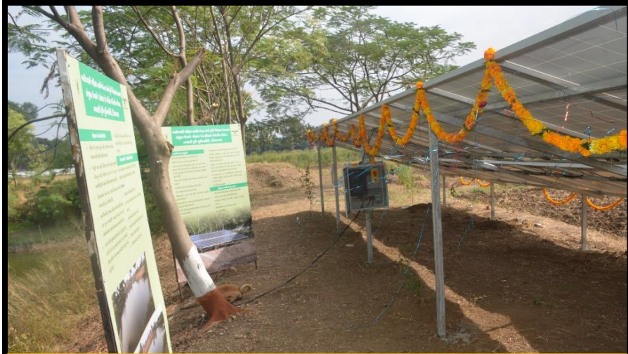
Solar Pump Demonstration Unit
